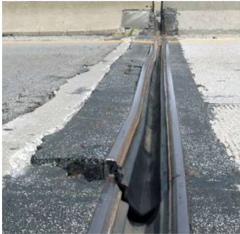
(a) Bridge expansion joint damaged David (2017).
