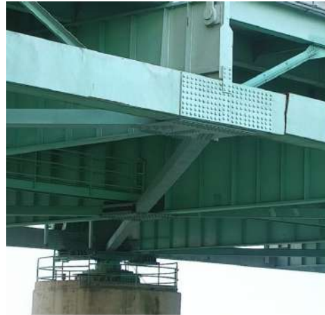
(b) Fatigue crack growth in steel beam Rob (2021).
